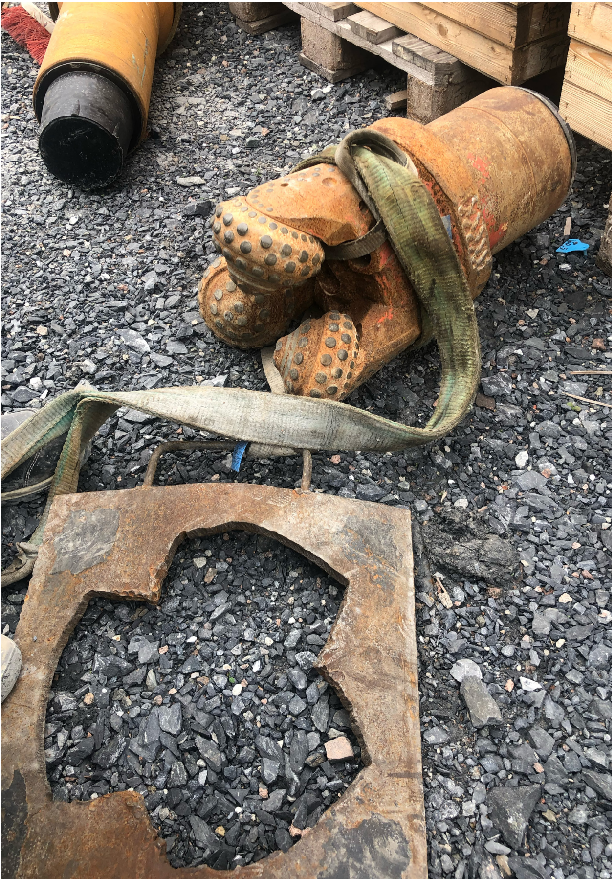
Seen on one of our visits to the building site. The object there is a drill bit they are using to dig a tunnel to the sea, as part of the energy system in the new museum.
