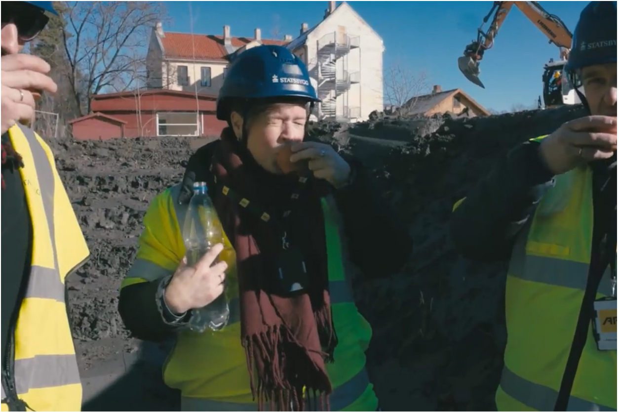
Henrik, Sigrid and Christian down in the construction hole drinking water from the ceramic cups.
